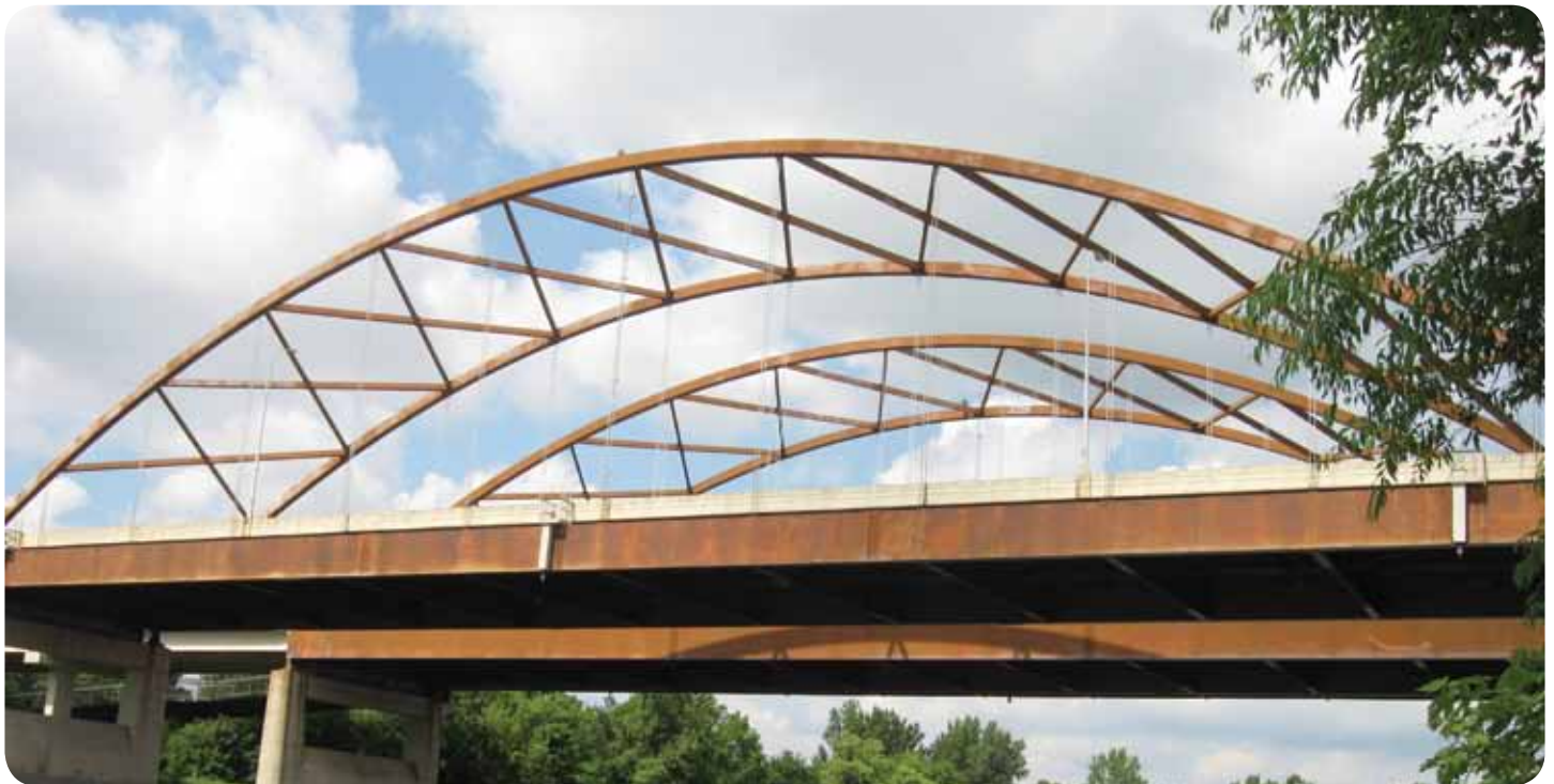
Acoustic sensors listen for potential problems—such as a bolt cracking—to monitor the health of a bridge.
