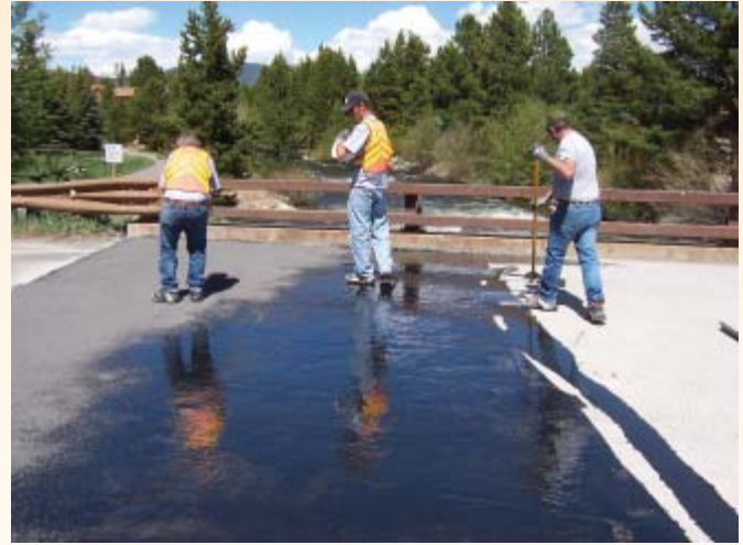
Fine taconite aggregate is applied over a tacky, adhesive base on a bridge deck in Frisco, Colorado. This pilot project tests Mesabi Hard Rock applications to reduce vehicle skidding on bridges.
