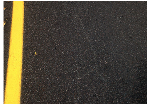
Microsurfacing project after two years: the start of underlying cracks through the surface layer
