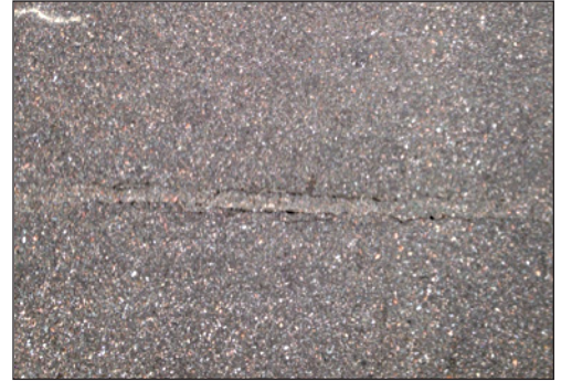
Microsurfacing project after two years: minor fatigue cracking
