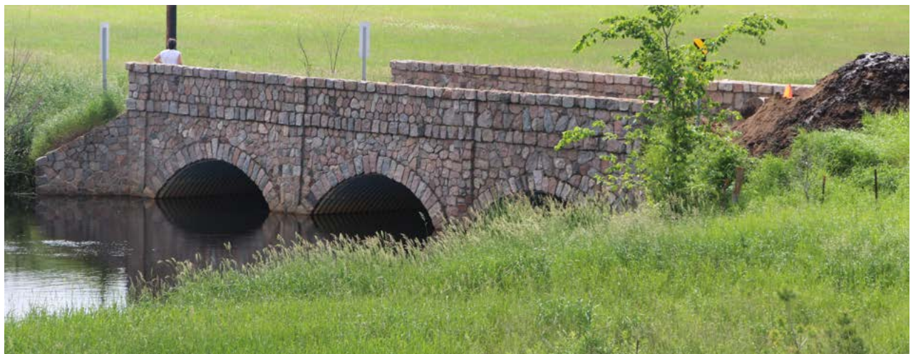
Todd County's multi-plate arch has a rock façade and early steel plate design.
