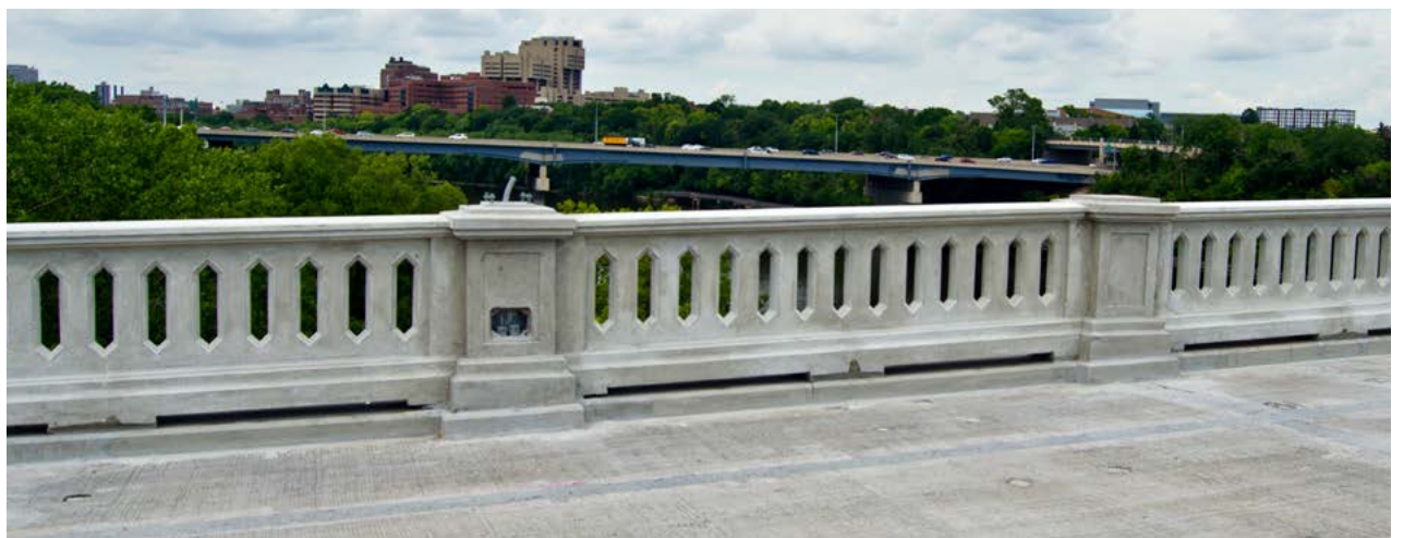
The new deck and substructure repairs of the Franklin Avenue bridge in Minneapolis respect the original design.
