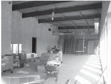
Construction of new general office space in the addition to the Cereal Disease Lab.
