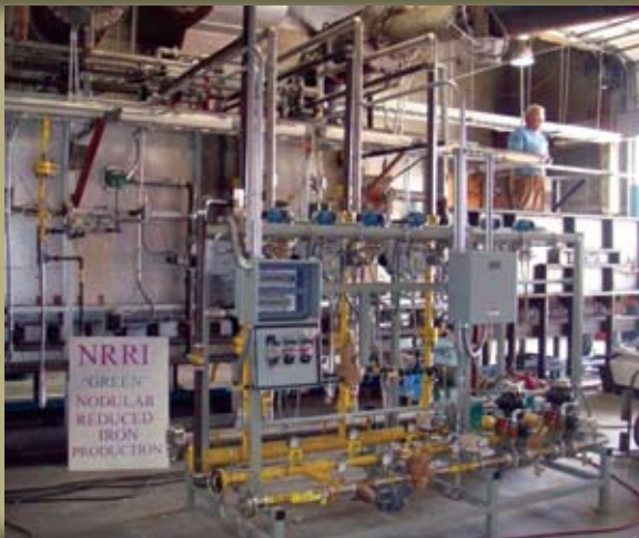
Pilot-scale iron nugget furnace with oxyfuel coal burners
