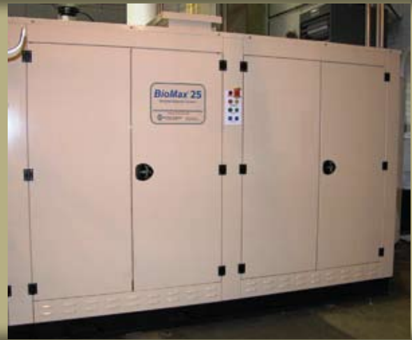
25 kW biomass gasifier
