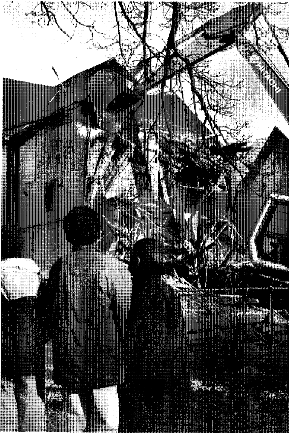
An abandoned house can become not only an eyesore but a hang-out for kids and a place for drug deals. Sometimes, the best solution is to tear it down. Instead of the year or more this usually takes, this house on Girard came down within months because of the coordinated efforts of officials working in the CARE committee.
