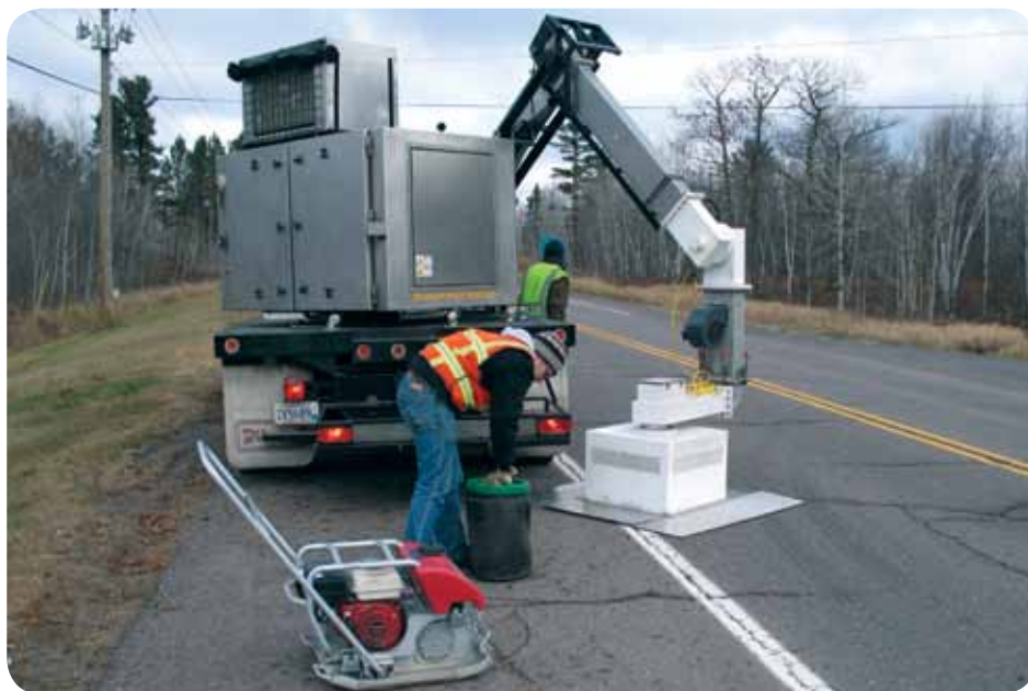
The microwave equipment is used to heat the pothole repair and surrounding pavement.
