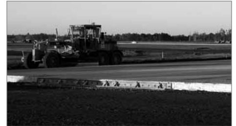
A runway construction project could be broken up into grading one year, followed by paving and final work the next.
