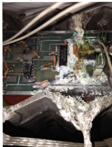
Fig 2 - A Corroded Preamp
