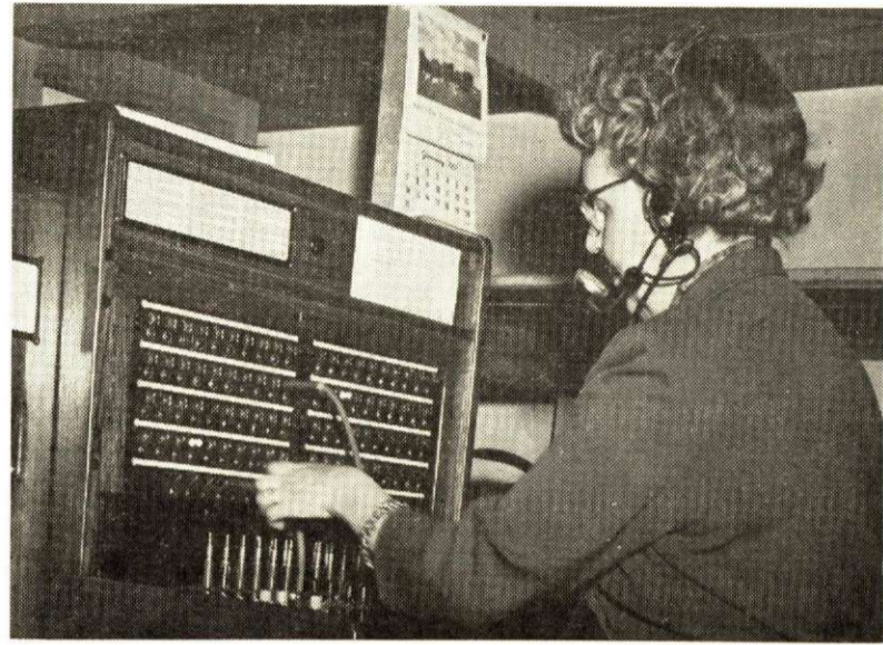
Operator Mrs. C. H. Alexander is shown completing a university call through the newly installed switchboard. —Photo by Hall
