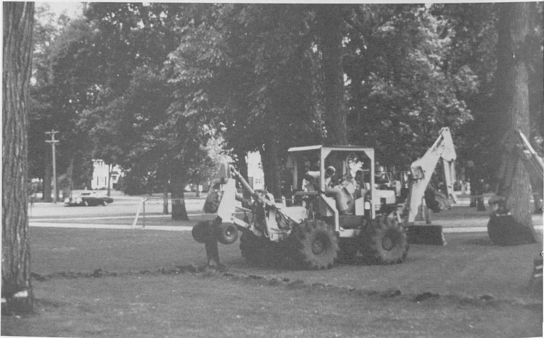
Figure 2. It is important to check for the presence of underground utilities before using a vibratory plow to disrupt root grafts.
