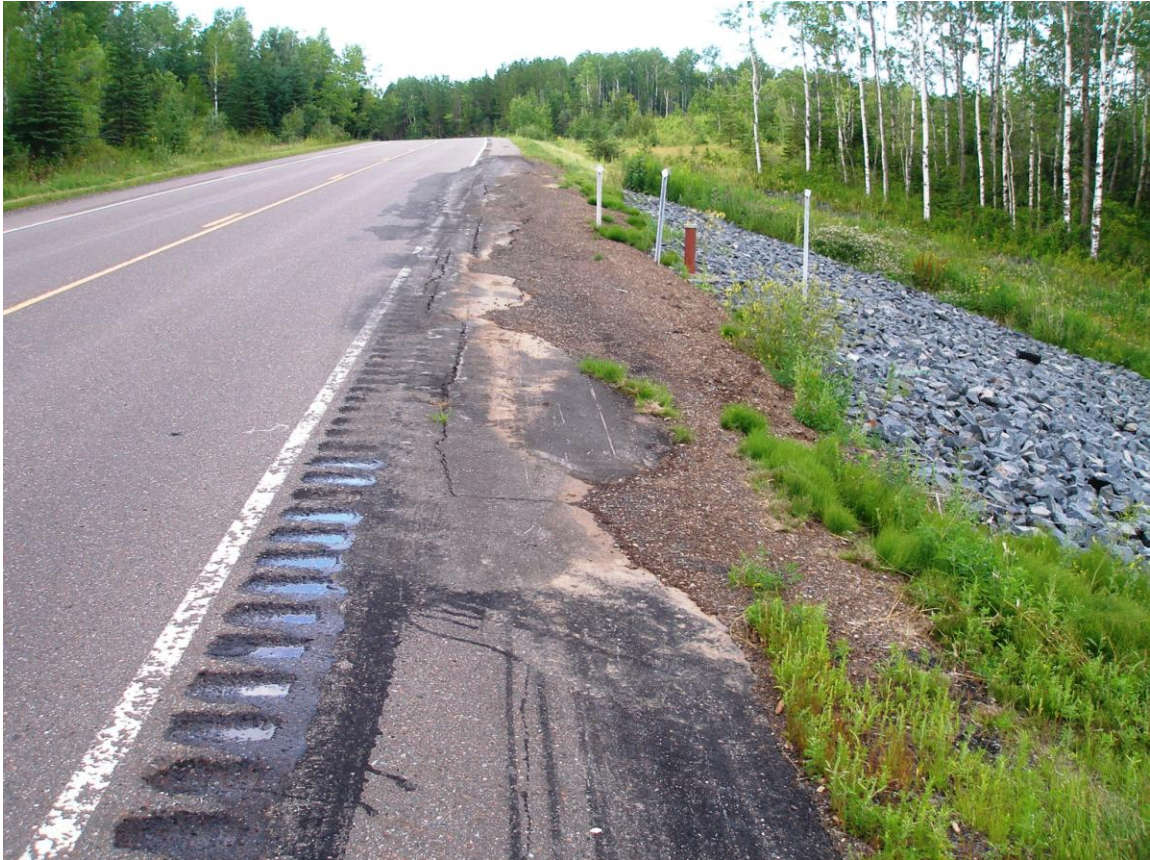
Figure 6. Repaired slump on Highway 23 at the South Fork of the Nemadji River.
