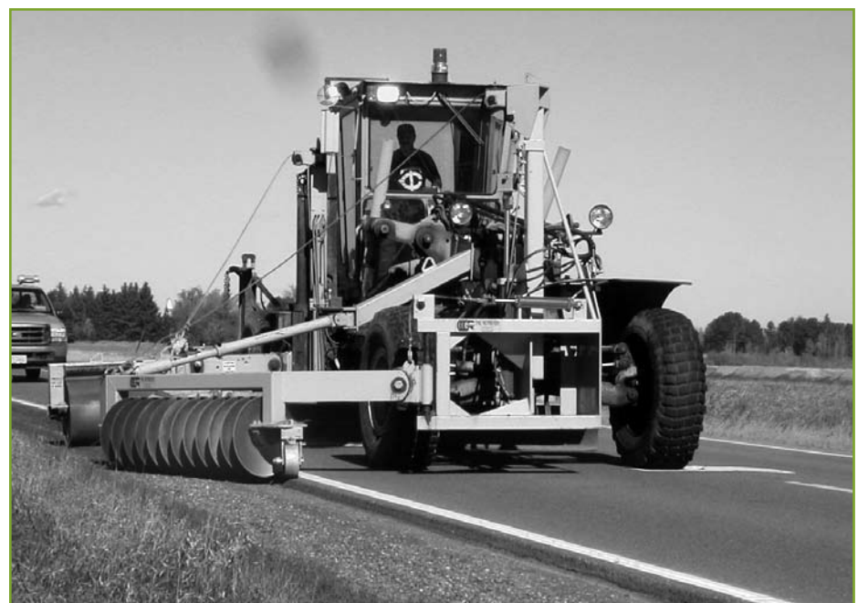
The unit reclaims material, and a vibrating roller levels it and packs it in place.
