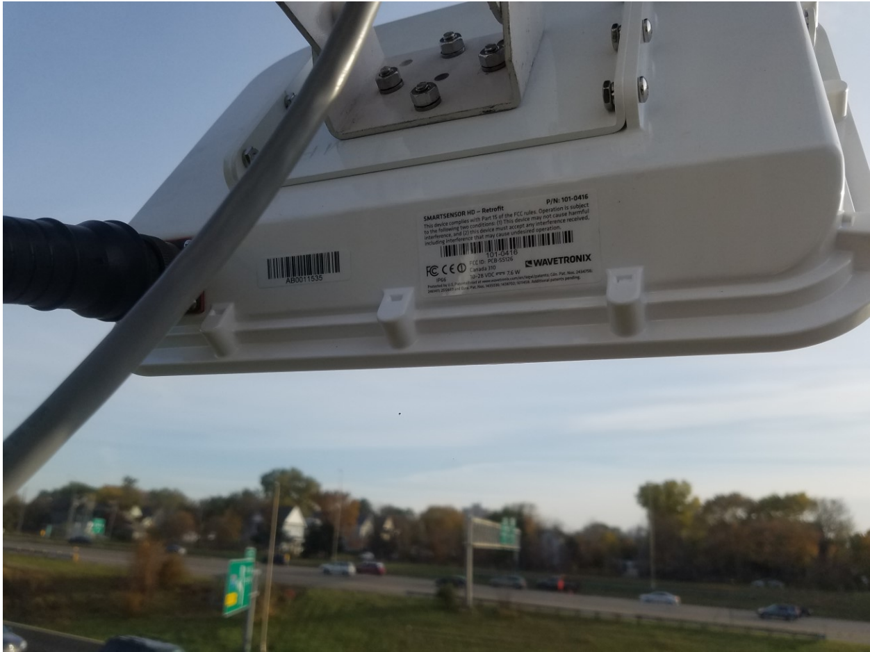
Figure 2.11 Close-up of Wavetronix sensor mounted at Hiawatha Ave.
