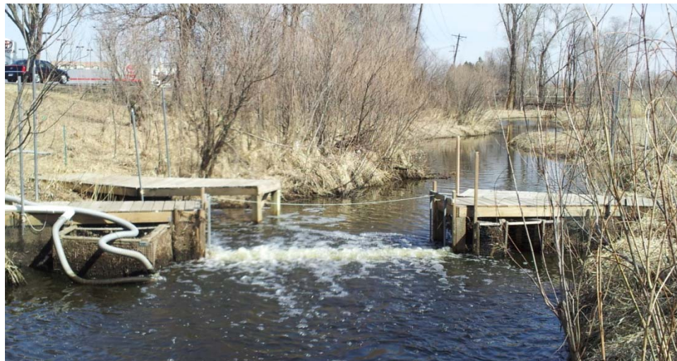
Figure 3-2. Plan view schematic of the bubble curtain system in Kohlman Creek with locations of release points for each movement test (top panel), and photograph of bubble curtain system and dock support structure, looking upstream (bottom panel). Photograph by author.
