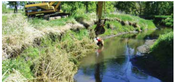
Stream restoration with boulders, willows and native plantings, Chankaska Creek - Kasota, MN
