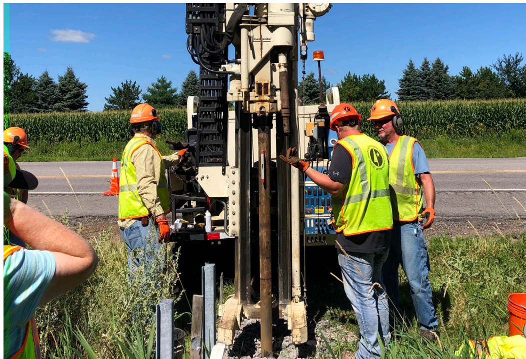
Near the end of the study, workers used a boring machine to take core samples of the ditch check and the filter insert.
