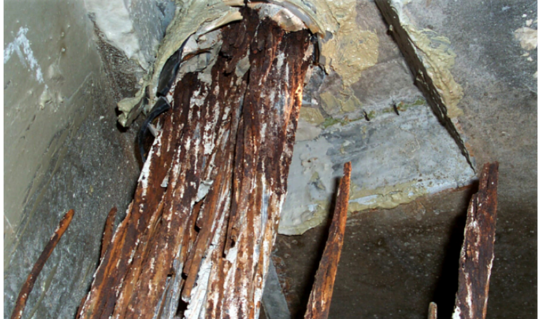
Figure 2.4 Corroded tendon found in Sunshine Skyway [30]
