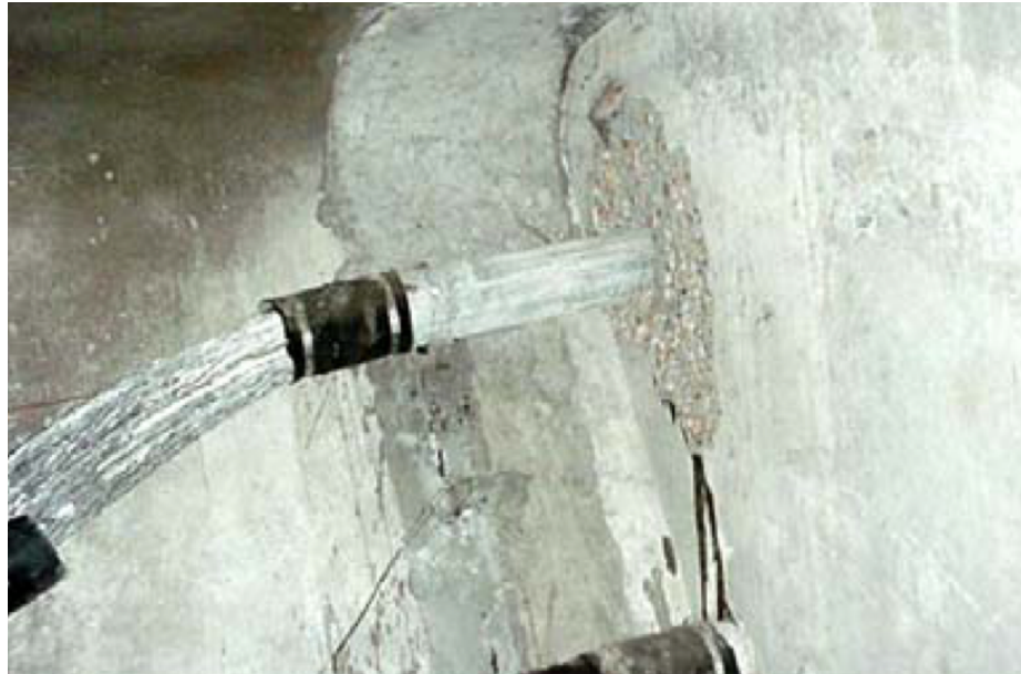
Figure 2.3 Midbay Bridge tendon failure [30]
