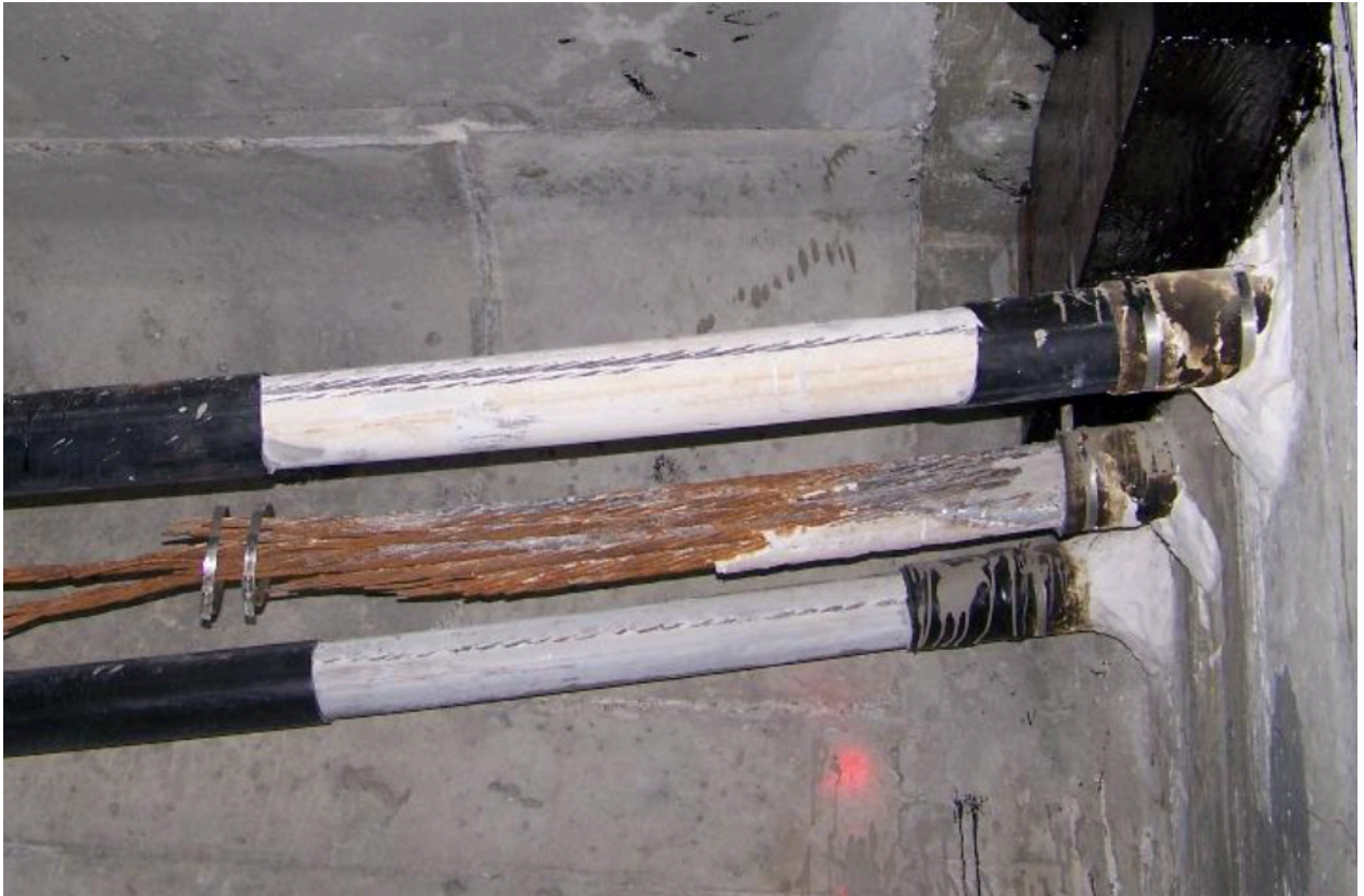
Figure 2.5 Corroded tendon from Verina Enon Bridge [32]
