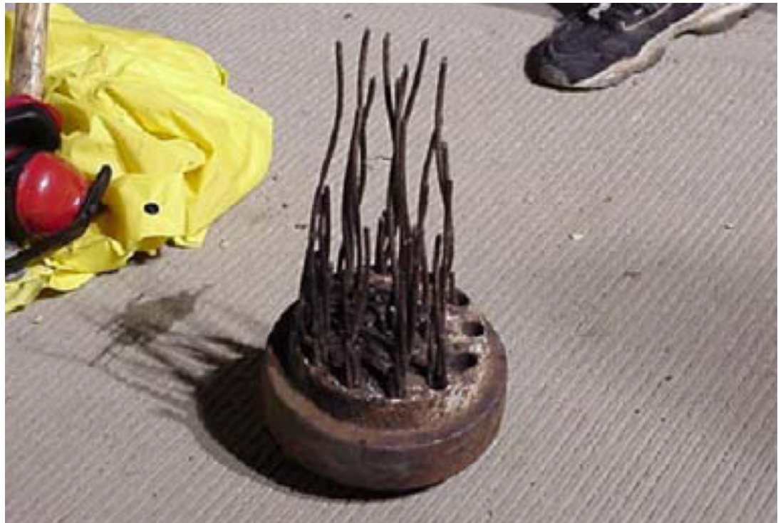
Figure 2.2 Corroded end-cap from a Niles Channel Bridge tendon [29]
