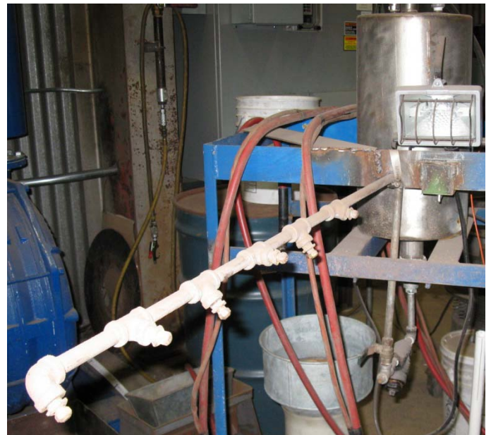
Figure 4 Granulation Drum Water Spray Bar
