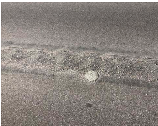
A mound of fill indicates where a test core was pulled from a joint that used J-Band.
