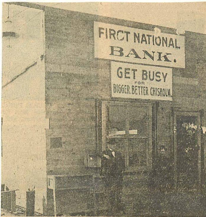
The First National Bank rebuilding after the fire. Gentleman in the door is Mr. G. L. Train, life long banker of Chisholm.
