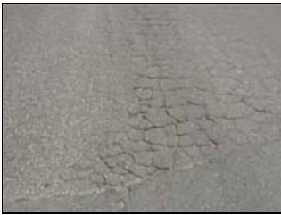
Pavement damage may result from poor subgrade drainage.
