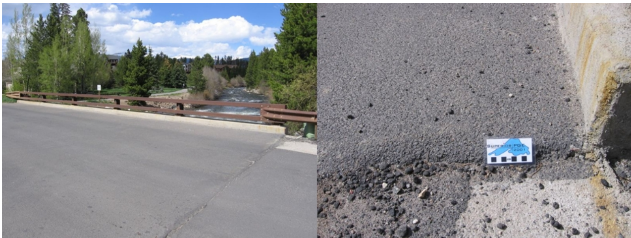
Figure 9. Frisco, CO, bridge deck one year after installation (left), and close-up of coarse taconite tailings used for friction course (right). Photographs taken on May 25, 2007.
