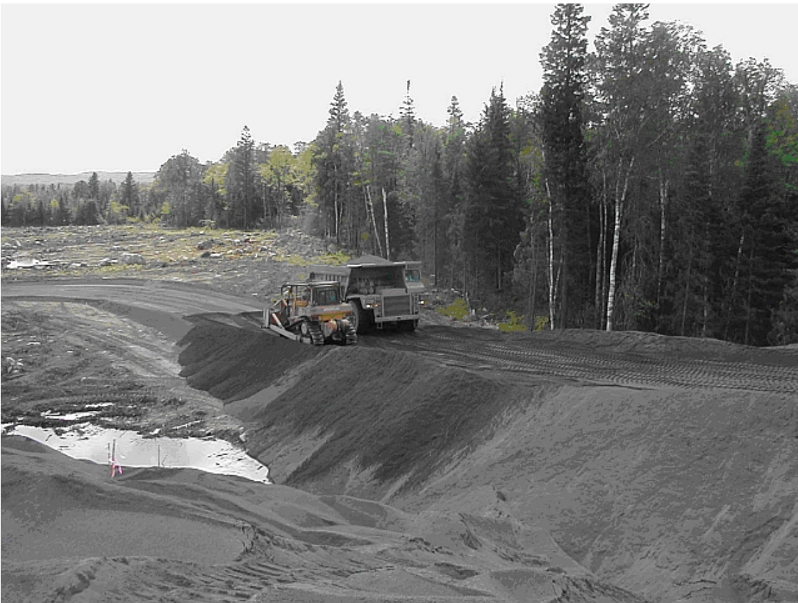
FIGURE 8 US TH53 / MN TH169 interchange construction north of Virginia. Photo by K. Adolfs.
