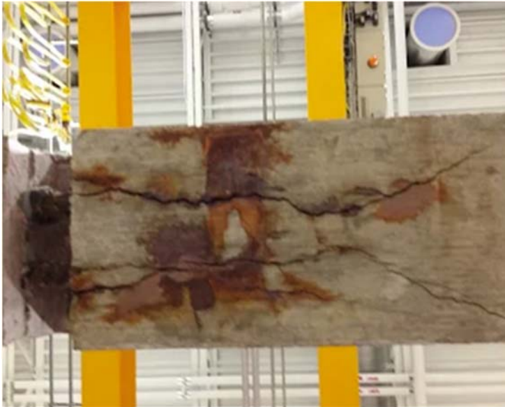
Deterioration of an RC beam due to corrosion
