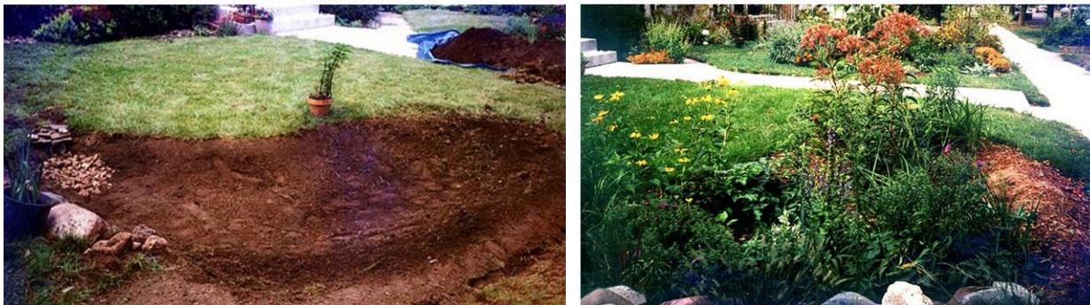
Fig 6. Residential rain garden A) under construction and B) completed. Photo by Mary Nolte.
