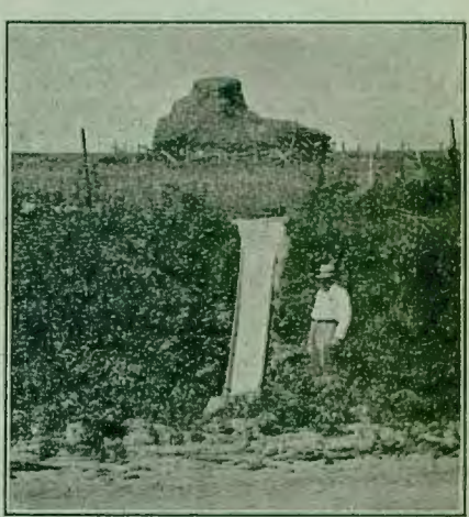
Fig. 2. Galvanized iron flume as terrace outlet. Fall about 10 feet. Location southeastern Minnesota
