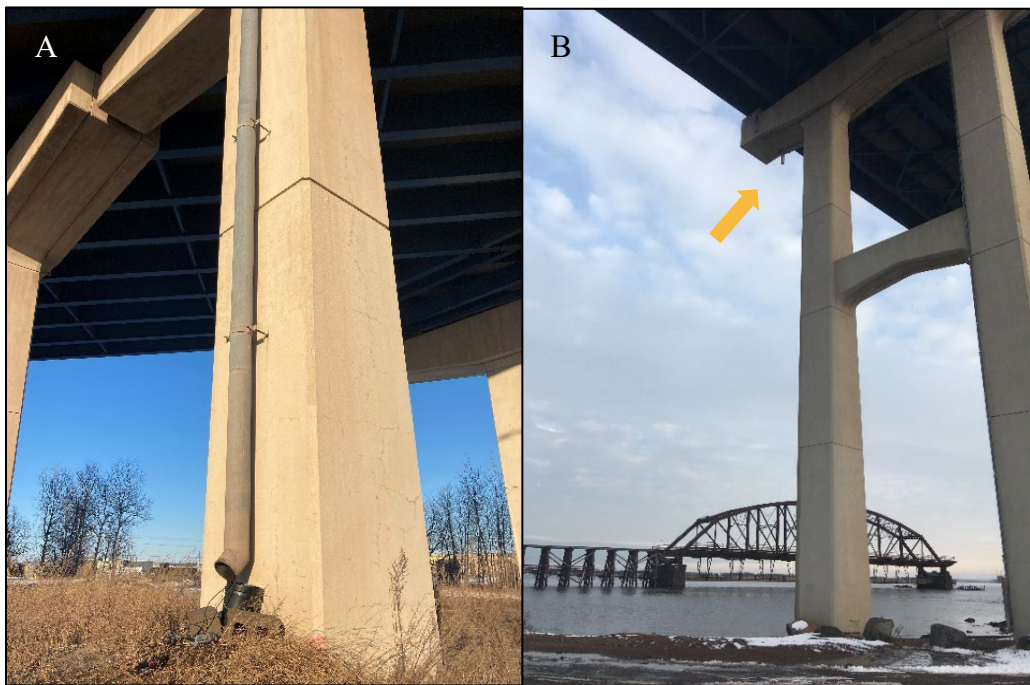
Figure 9. (A) BB-KAc-B; with the collection bucket; (B) BB-RP-B, with an arrow pointing to the discharge pipe over the sampling location
