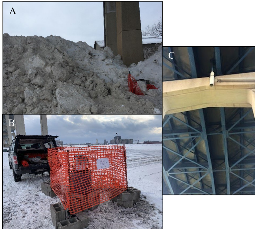
Figure 8. Bridge runoff collection sites at Blatnik Bridge: (A) initial runoff site, (B) current runoff site, and (C) second drainage pipe, drops water into picture B
