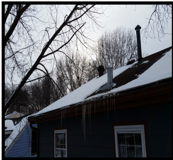
Image 4: Snowmelt pattern in middle of roof indicates uneven heating of the roof deck. This was theorized to be an area where heat leakage was rather high from the house.
