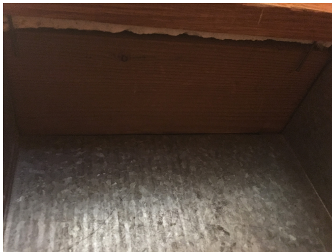
leaking into the attic
