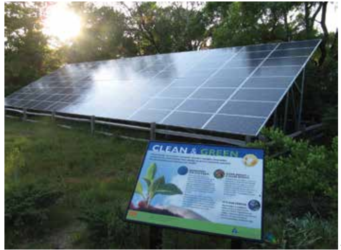
Figure 4: Sign explaining conversion to solar energy.
