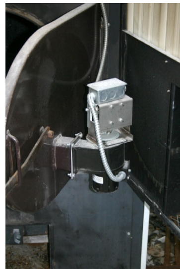
Figure 8- A close-up of the parts that were added to the gasifier
