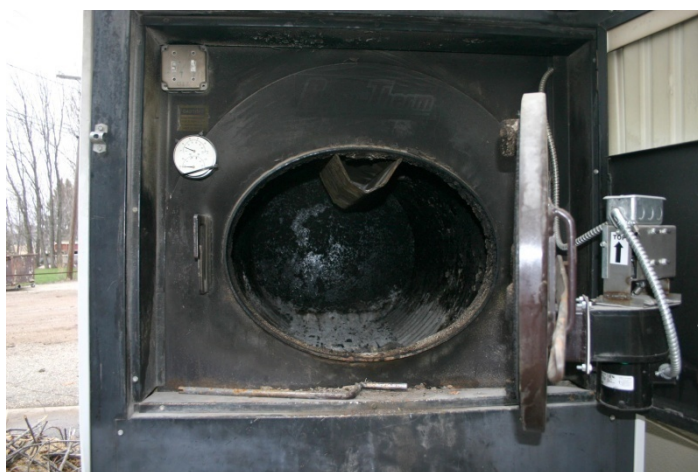
Figure 6- Picture of the Wood Burner and the gasification parts that were installed.
