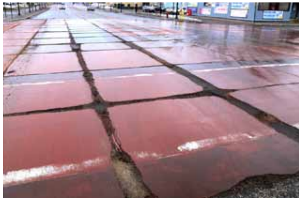
Fig. 6: Early distress in colored concrete in Centerville, MN
