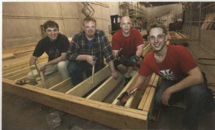
Construction management students Bradley Fasbender, Clayton Tallman, Matt Klemmensen, and Grant Gardener (left to right) take a break from constructing the foundation at the University's ReUse Center.
