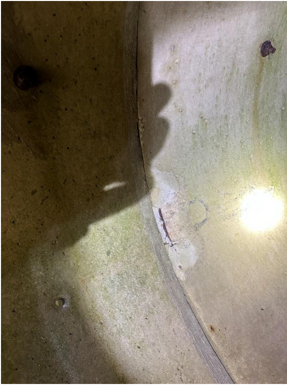
(c) Culvert 2187828, District 6: 2-in. separation on joint with exterior pipe ties
