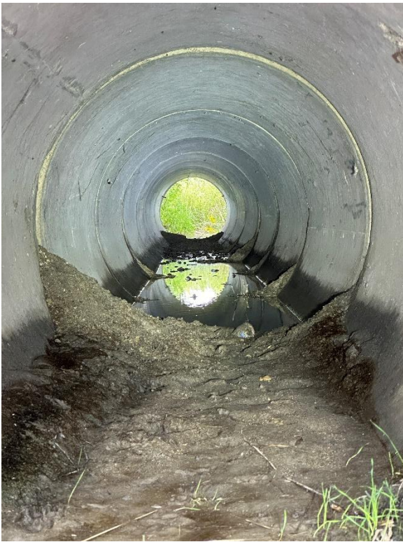
(a) Culvert 2251008, District 8: Some separation and infiltration at all joints
