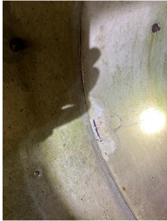
(d) Culvert 2196332, Metro District: 6-7 in. of separation, breakage of joint
