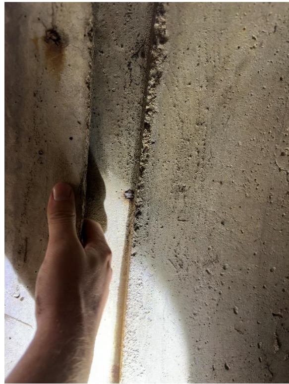
(b) Culvert 2251023, District 8: 3 in. separation at first joint
