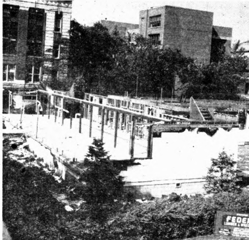
Ribs protruding, former temporary south of Vincent (Mrs. Murphy) faces its last days of existence. Workmen should have the building completely removed from the site by Thursday, according to H. L. Wilson, physical plant engineer. Contractors will begin work on the erection of Ford hall, the new social science building, immediately afterward, Wilson said.
