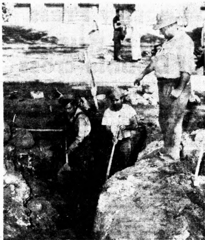
MOVING STORM SEWER DRAINS in front of Westbrook hall, Christ Arne, left, and Quinn Wellington, center, are directed by Clarence Carlson, foreman. The job is part of moving Fifteenth avenue S.E. to make room for a new classroom building which will be built where temporary north of Library now stands. The new street should be completed by the beginning of fall quarter, Carlson said yesterday.
