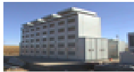
Figure 1.7: Xcel Energy battery facility
