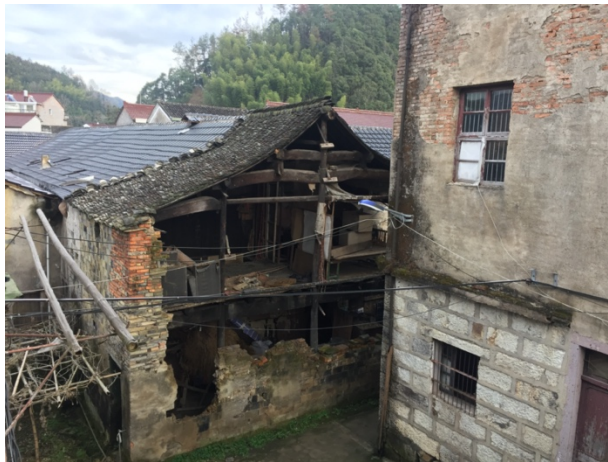
Figure 1: A broken house in Red Mountain Township
