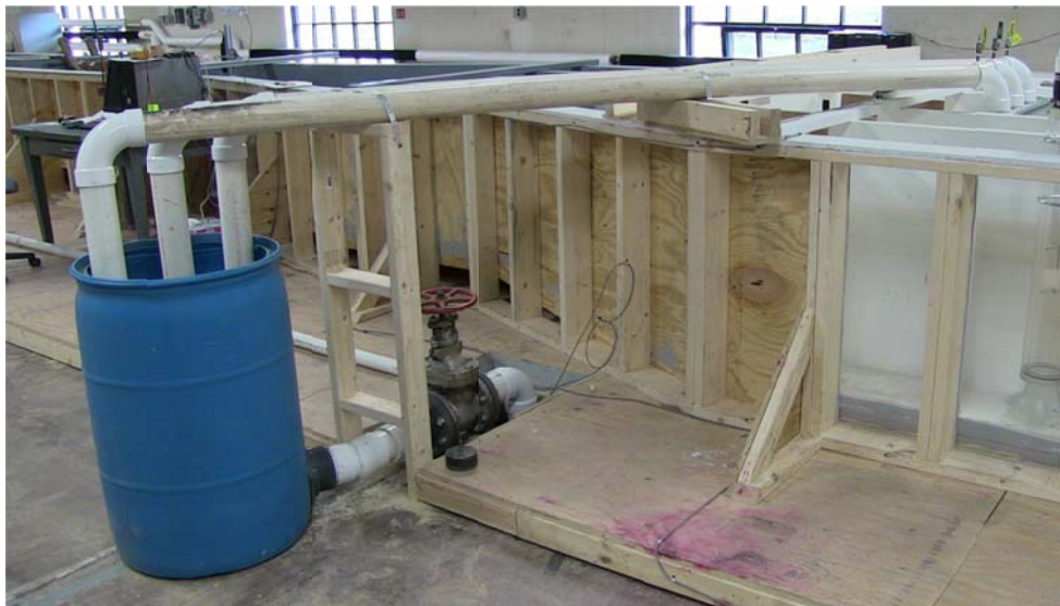
Figure 5: Combined Submersible Pump Discharge Plumbing
