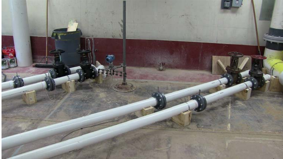
Figure 4: Vertical Turbine Pump Discharge Plumbing
