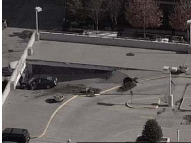
(a) Partial collapse
