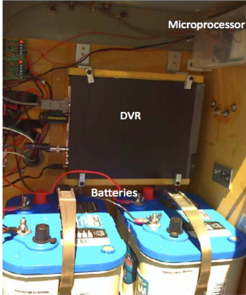
Figure 3: Inside of cabinet (batteries, DVR and microprocessor)
