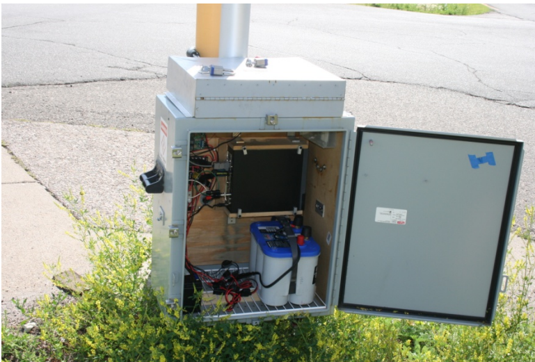
Figure 2: The cabinet with mounted components
