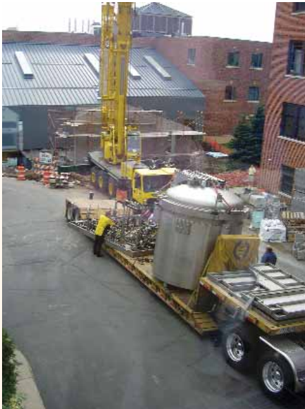
The chemical cremation waste-disposal system was installed and operational in early 2005.
