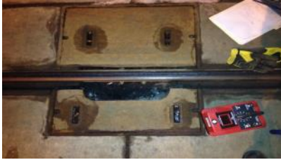
Rail Access Box
