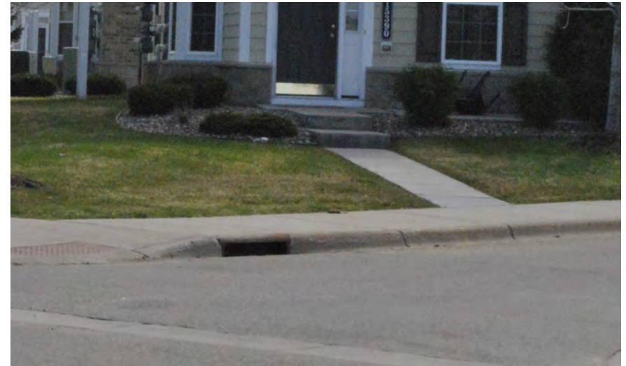
Unstenciled storm drain in Central Village, Apple Valley, MN
