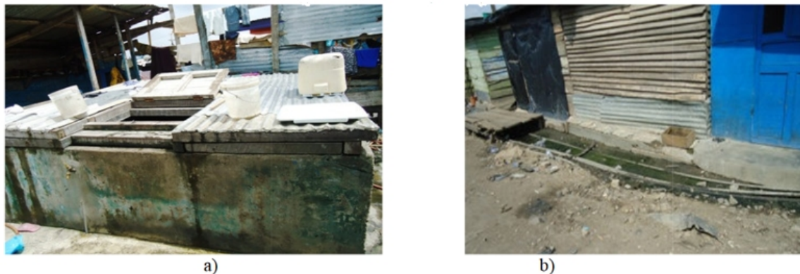
Figure 3.3: Concrete Water Tanks and Old pipelines in Accra, Ghana
