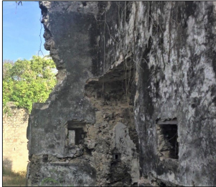
Figure 5.22: Interior of space 105 looking at entrance to north tower demonstrating lack of seaming and integration of door lintel into stonework.
