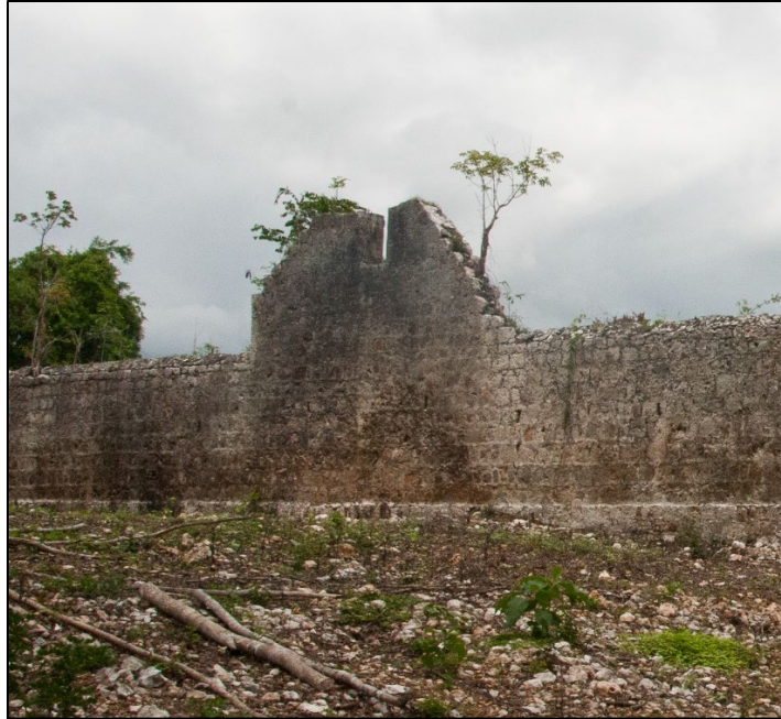
Figure 5.26: Detail of Courtyard east wall connection to structure 2, showing lack of seaming.
