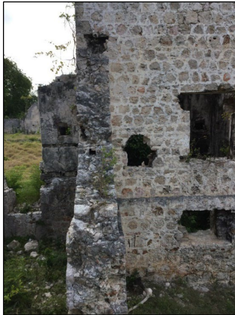
Figure 5.20: West façade of south tower demonstrating stone coursing and integration of structural framing.
