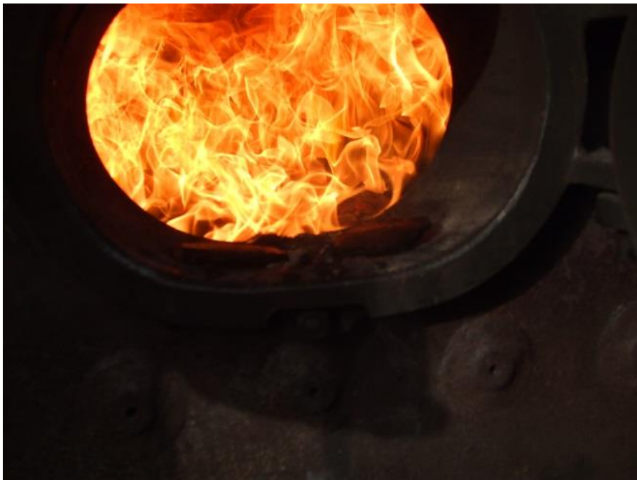
Figure III-9: Combustion of fuel briquettes under full draft conditions.
