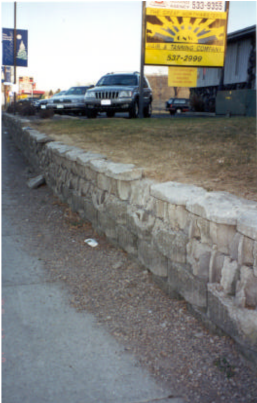
Figure 4.10. Overall photo of SCBRW subjectively rated as “very poor”.
