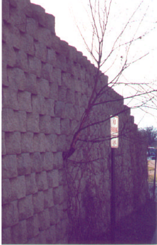
High-Severity Embedded Vegetative Growth
