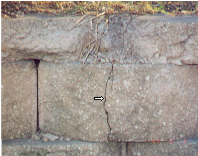
High-Severity Cracked Block
