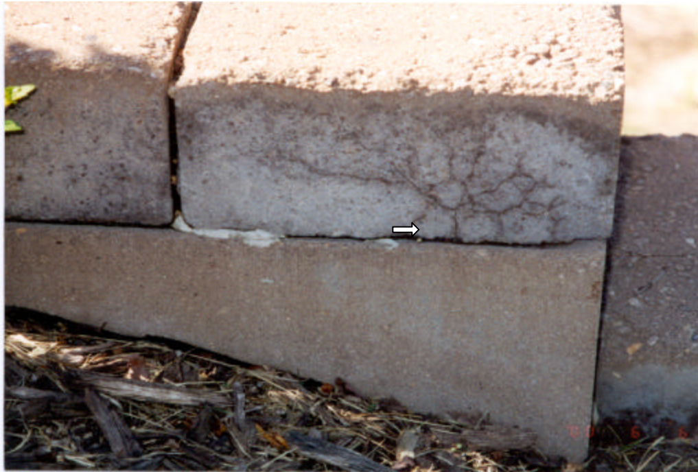
a. Medium-Severity Freeze-Thaw Damage (Top Block Layer).
