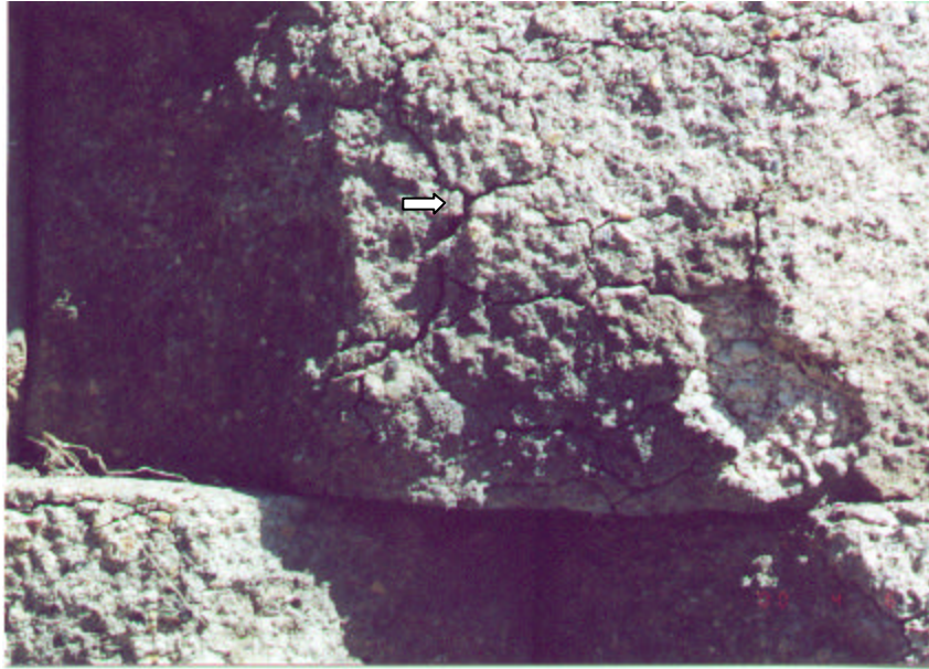
High-Severity Vertical Surface Freeze-Thaw Damage
