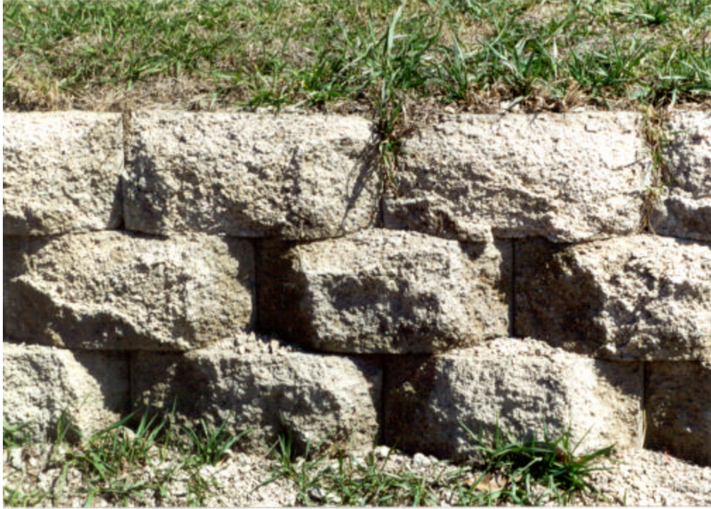
Figure 3.2. Close-up photo of northern portion of south wall (CSAH 101 and 24 th Ave.).
