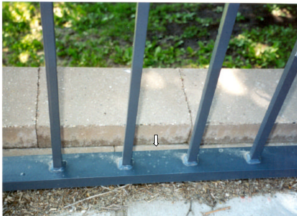
b. Low- and Medium-Severity Freeze-Thaw Damage (Top Block Layer).
