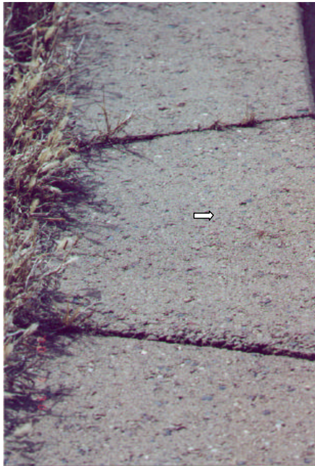
Low-Severity Top Block Layer Scaling
