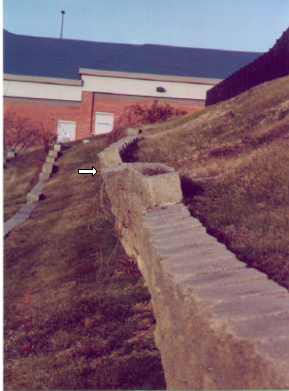
High-Severity Structural Distress
