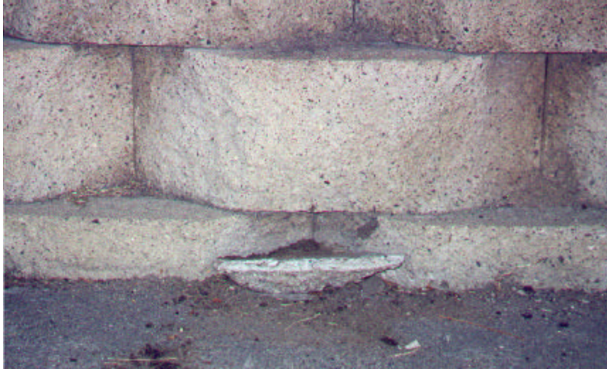
Bottom Block Popped out of Ground.
