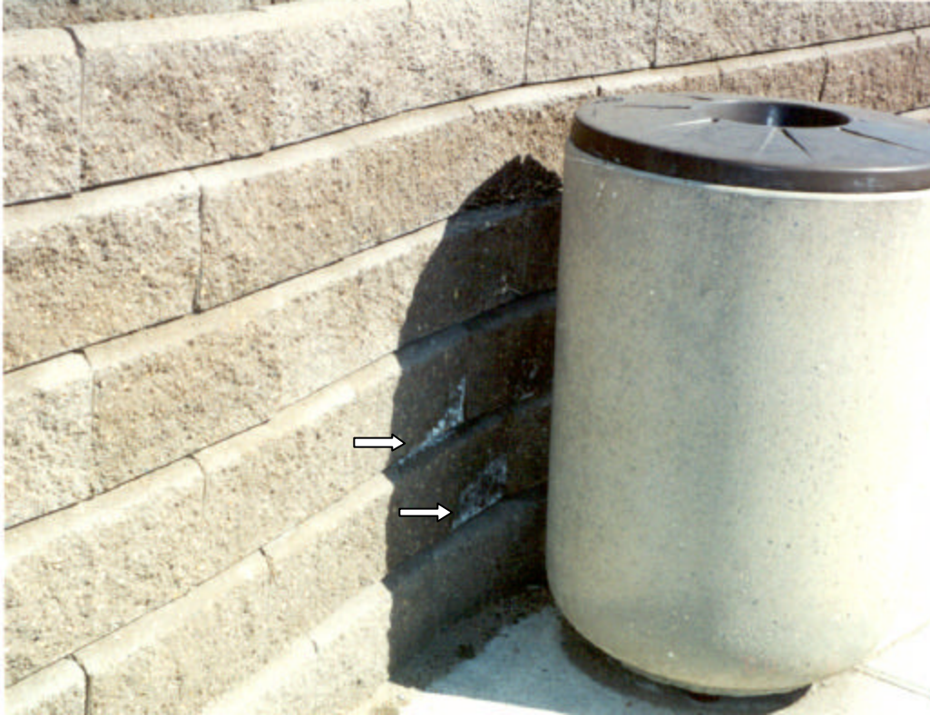
a. Efflorescence behind obstruction.
