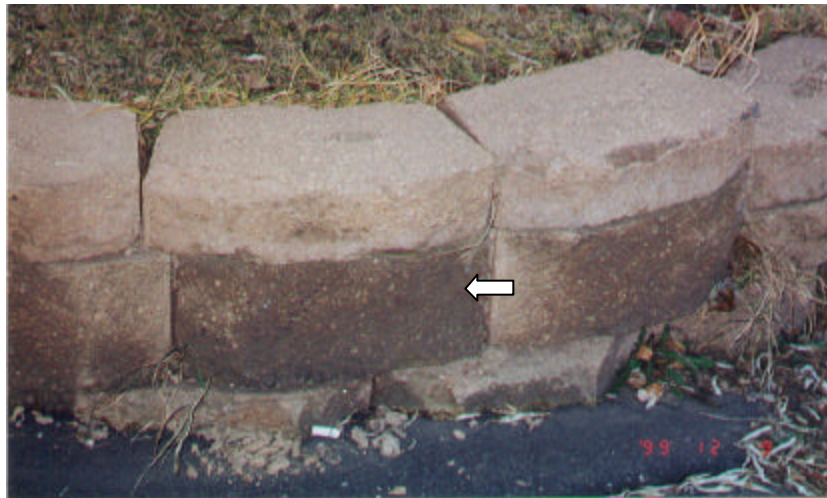
High-Severity Staining (External Source)
