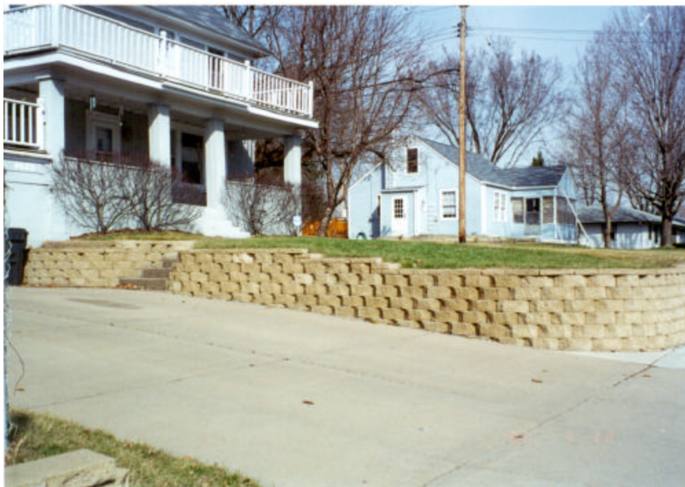
Figure 4.26. Overall condition photo of SCBRW located in driveway subjectively rated as “good”.
