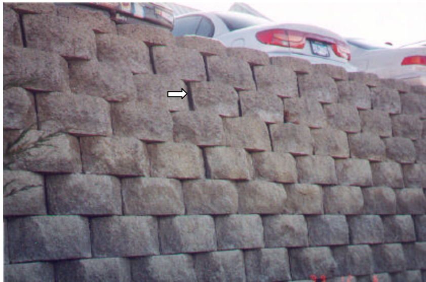
Medium-Severity Construction Flaw (Twisted Blocks)
