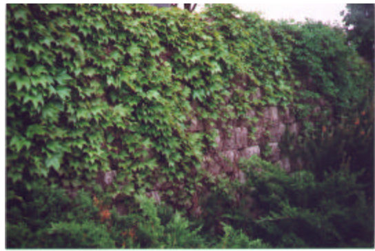
Medium-Severity Embedded Vegetative Growth
