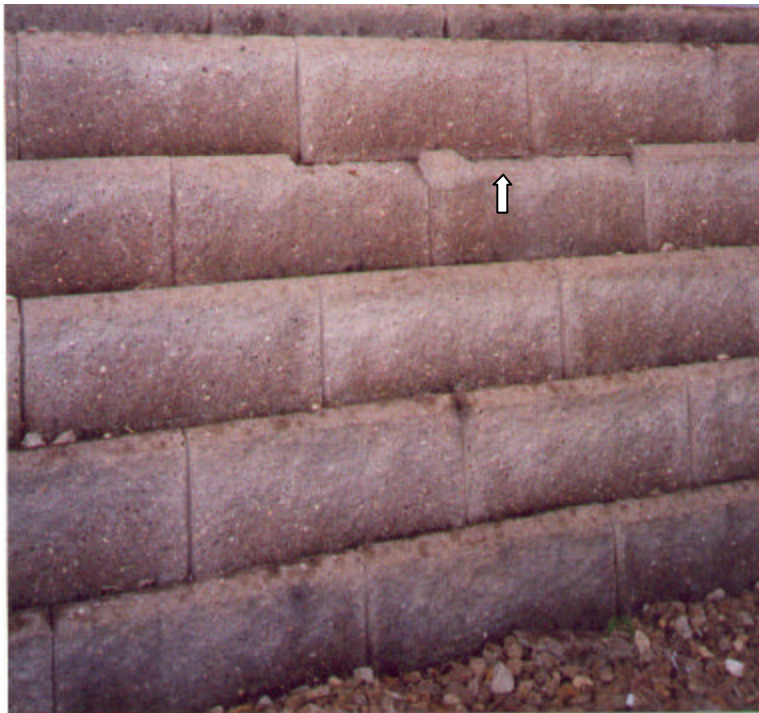
High-Severity Block Position Guide Damage
