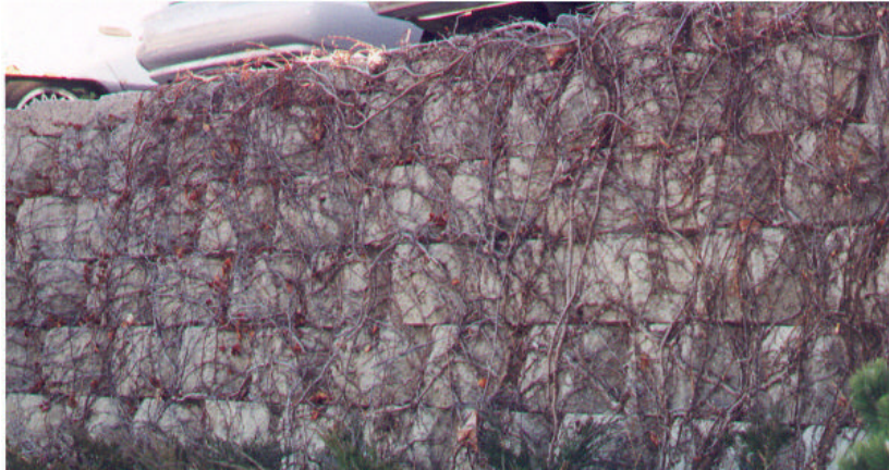
Medium-Severity Embedded Vegetative Growth
