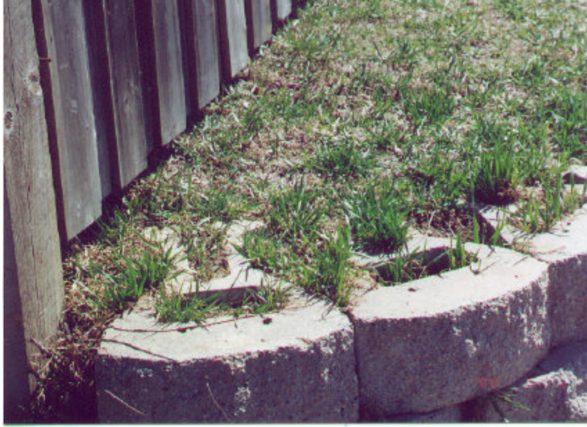
Missing Backfill behind Top Block Layer
