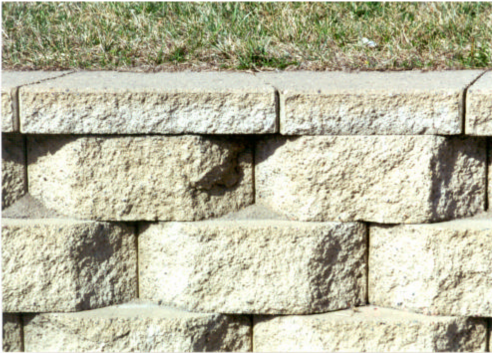
Figure 4.28. Photo of low-severity freeze-thaw damage on SCBRW subjectively rated as “good”.
