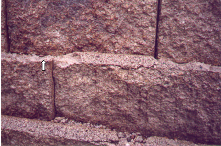
High-Severity Block Position Guide Damage
