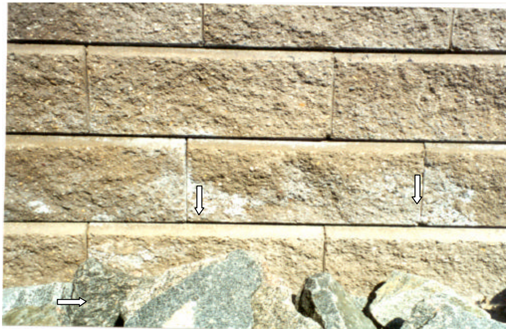
a. Efflorescence on blocks adjacent to water level of river.
