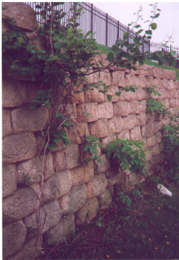
High-Severity Embedded Vegetative Growth
