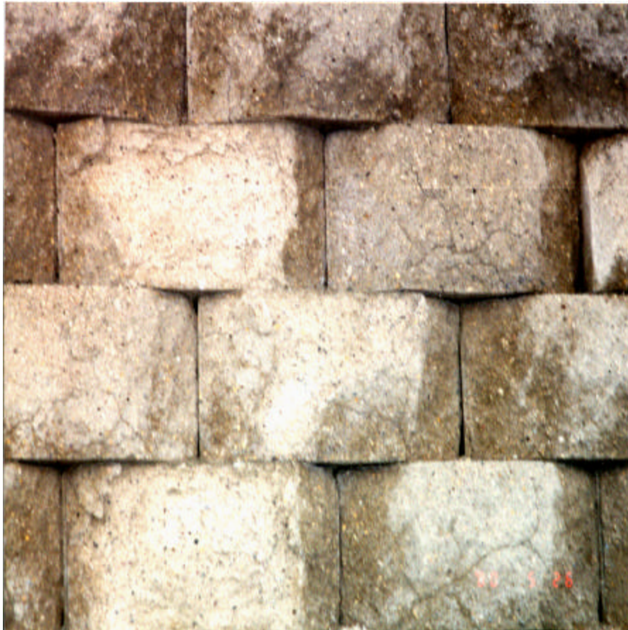
Figure 4.16. Close-up photo of high-severity scaling and high-severity freeze-thaw damage on SCBRW subjectively rated as “poor”.
