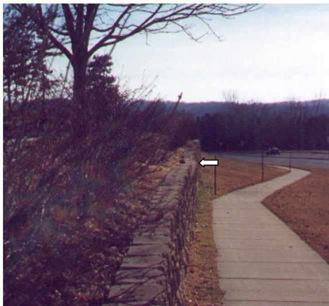
Low-Severity Structural Distress
