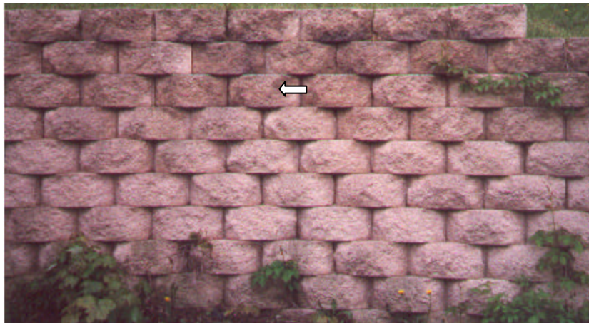
Medium-Severity Staining (External Source)
