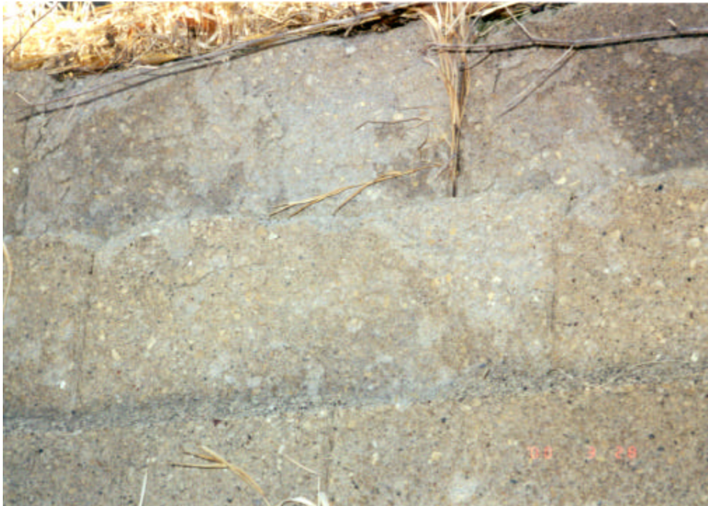
Figure 4.21. Close-up photo of high-severity scaling on SCBRW subjectively rated as “fair.”
