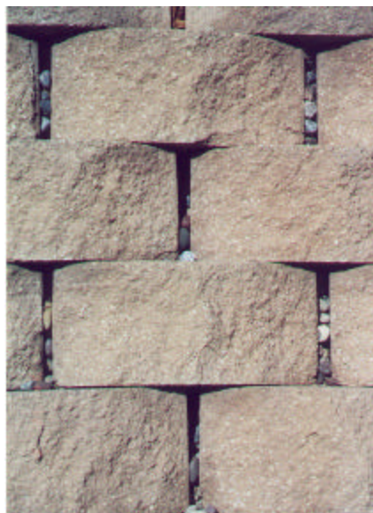
Medium-Severity Open Joints
