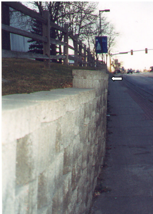
Medium-Severity Structural Distress
