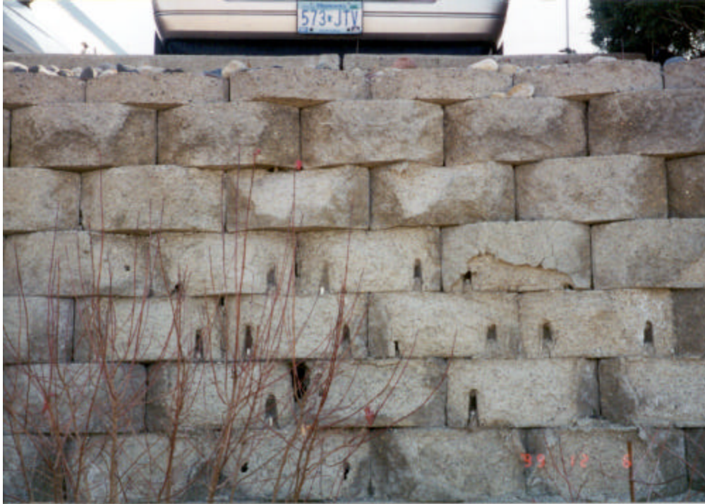
Figure 4.15. Close-up photo of high-severity scaling on SCBRW subjectively rated as “poor”.
