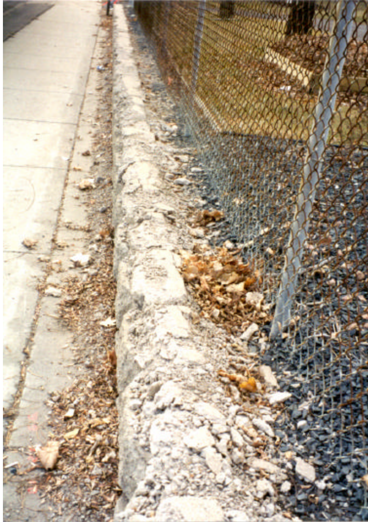
Figure 4.33. Photo illustrating high-severity freeze-thaw damage (top block layer) for wall with F/C distance of 8 ft.
