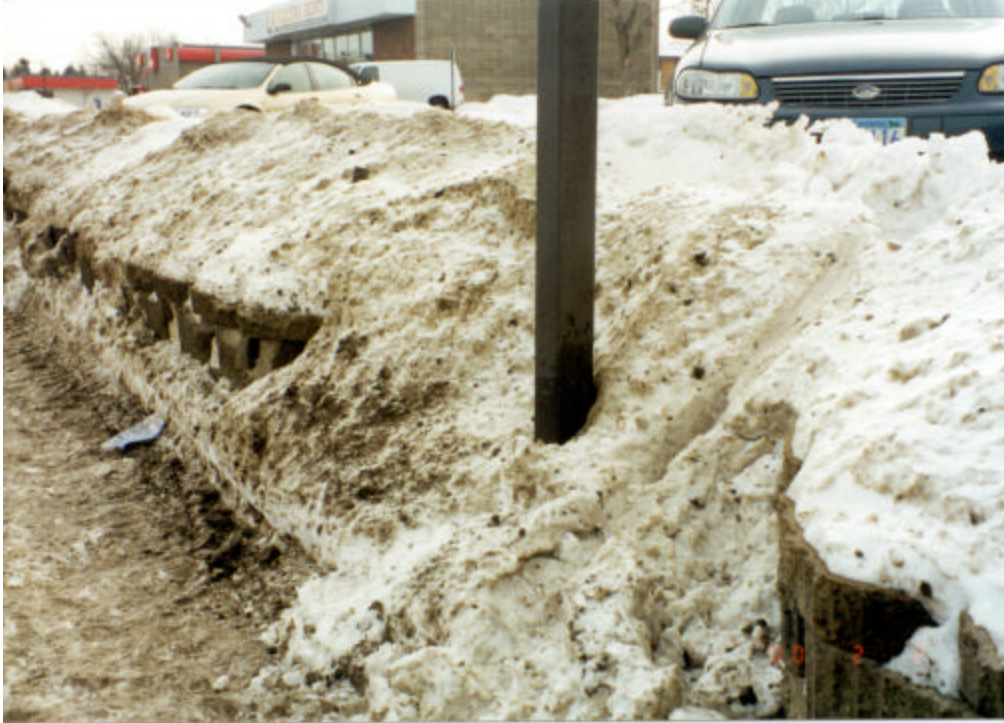
Figure 4.8. Photo of snow accumulation on curved segment of SCBRW subjectively rated as “very poor”.
