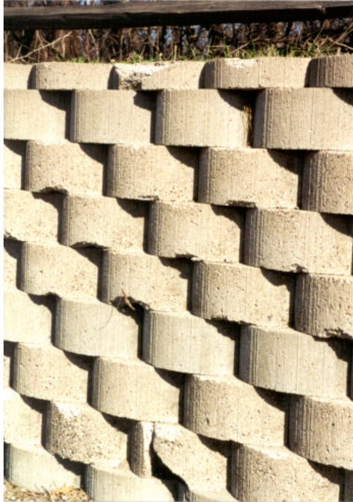
Figure 4.53. Durable and non-durable layers (CSAH 6 and 481 ft East of Dunkirk (north side)).
