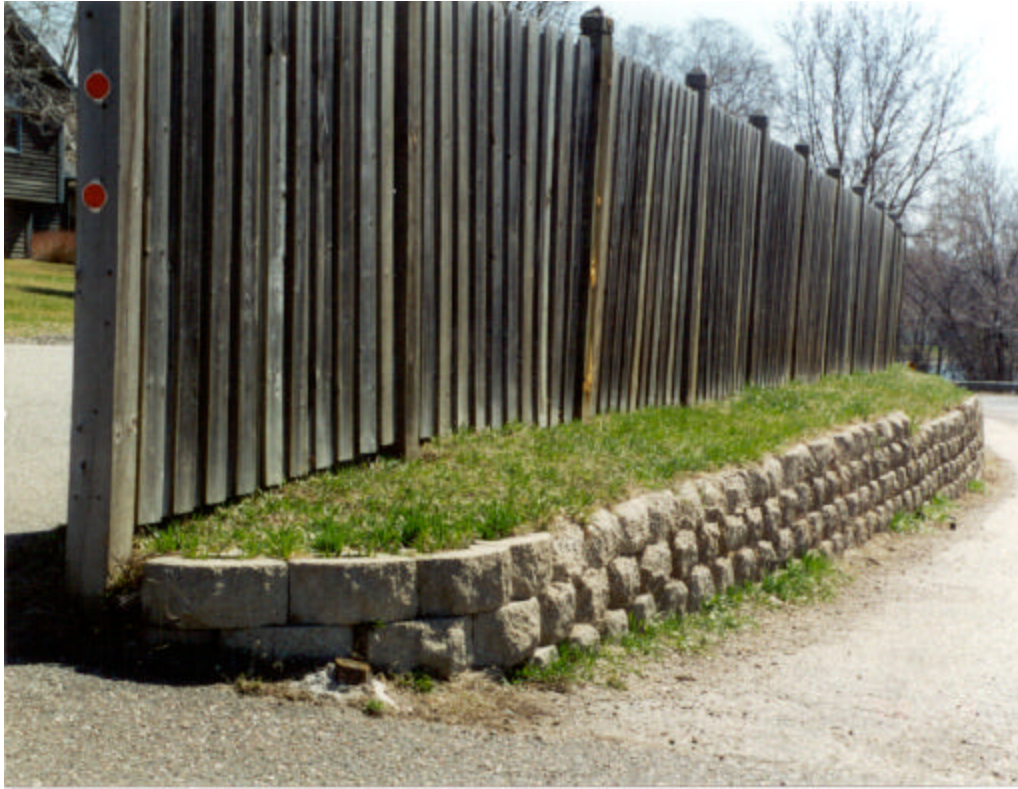
Figure 3.1. Overall photo of northern portion of south wall (CSAH 101 and 24 th Ave.).
