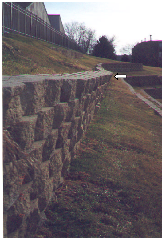
High-Severity Structural Distress
