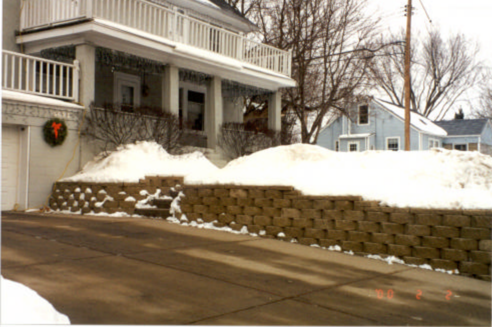
Figure 4.23. Photo of snow accumulation on portion of SCBRW located in driveway subjectively rated as “good”.
