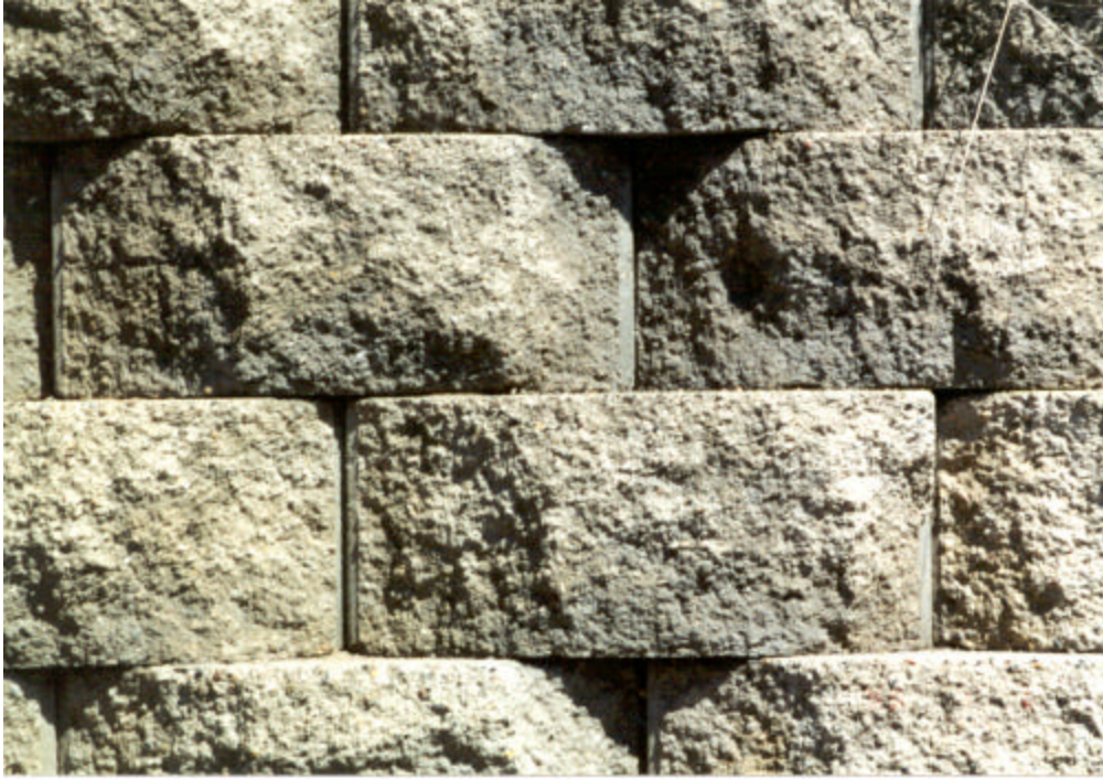
Figure 3.4. Close-up photo of southern portion of south wall (CSAH 101 and 24 th Ave.).
