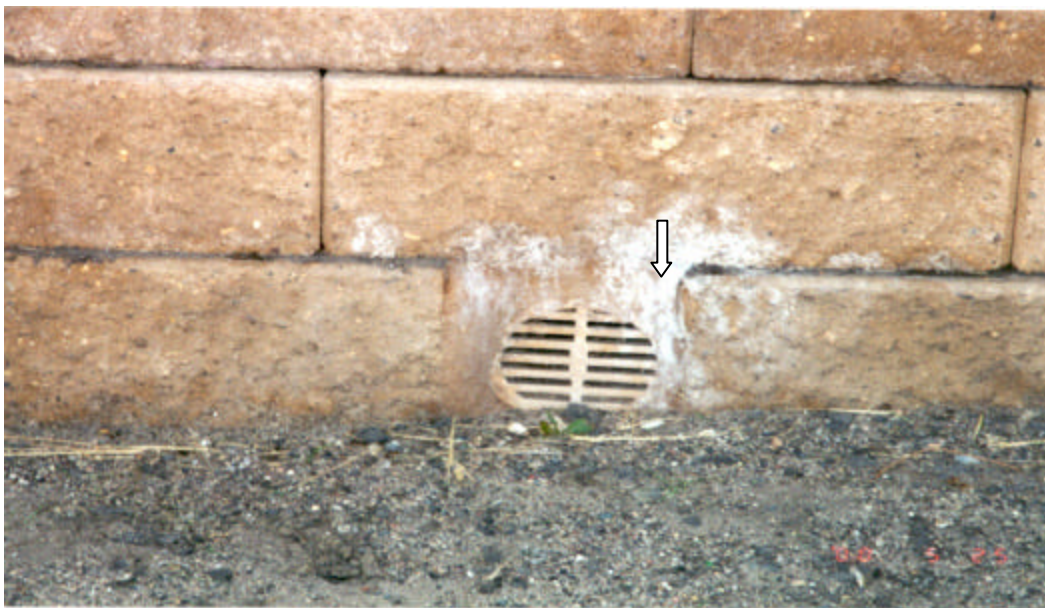
b. Efflorescence around drainage pipe.
