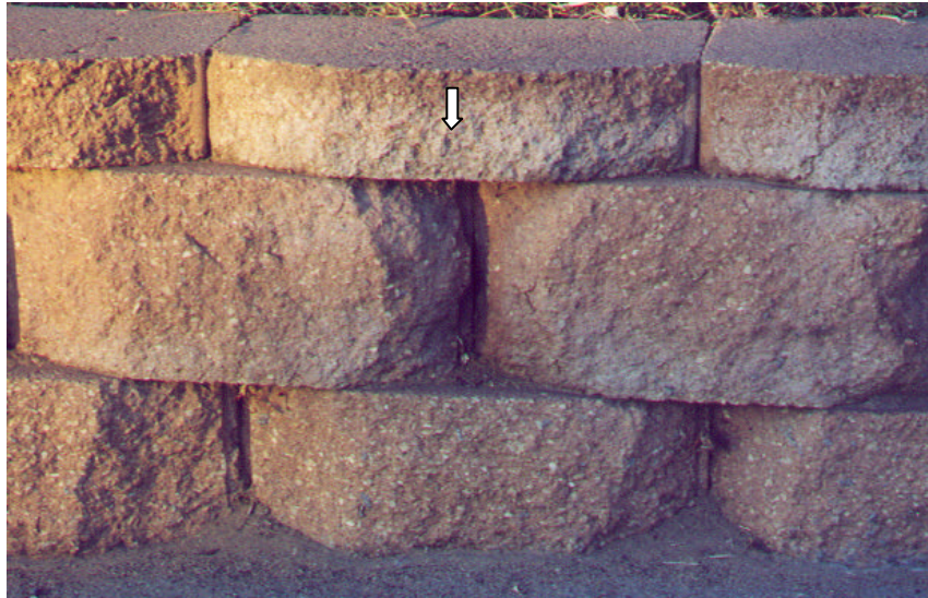
Low-Severity Capstone Freeze-Thaw Damage
