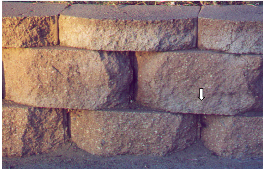
Low-Severity Vertical Surface Freeze-Thaw Damage
