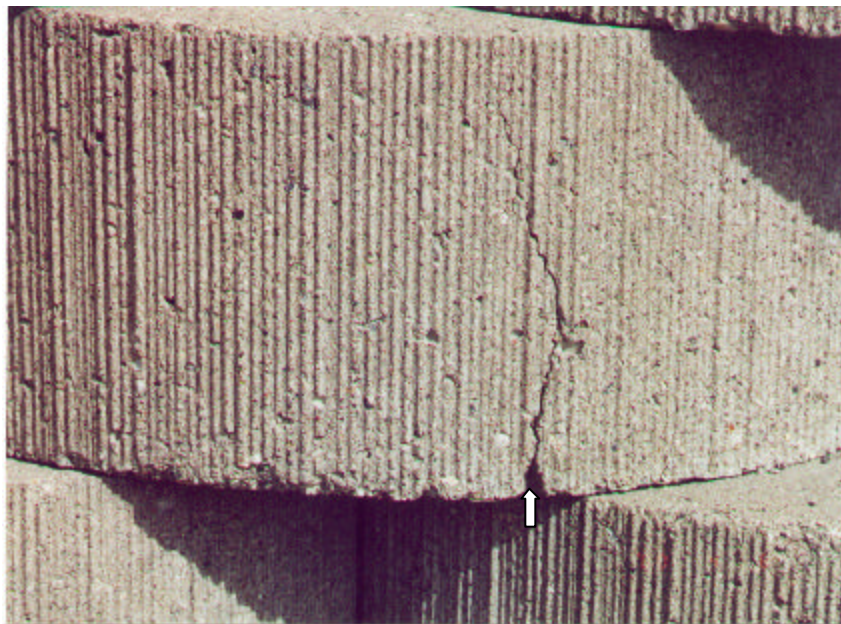
Low-Severity Cracked Block
