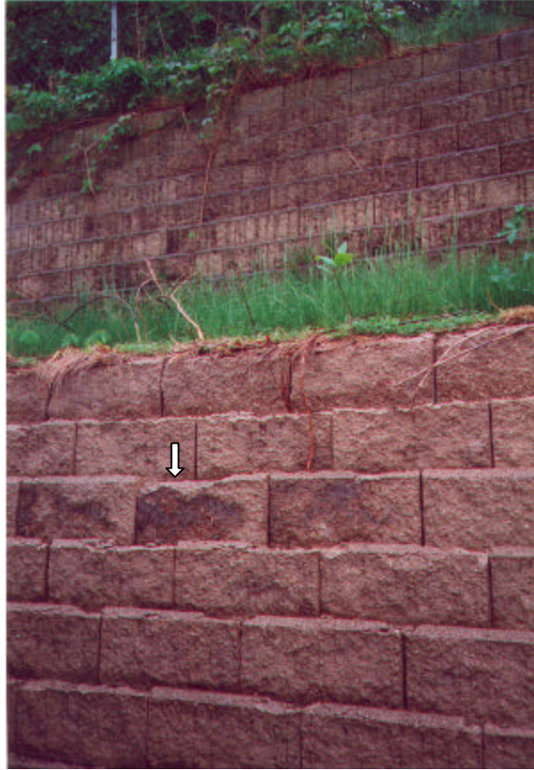
High-Severity Block Position Guide Damage
