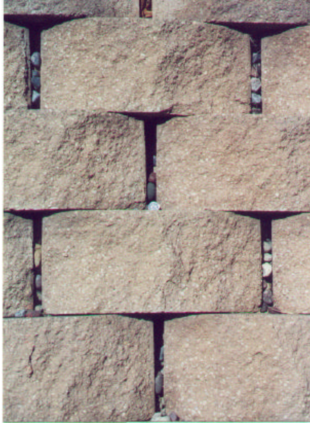
Medium-Severity Construction Flaw (Open Joints)
