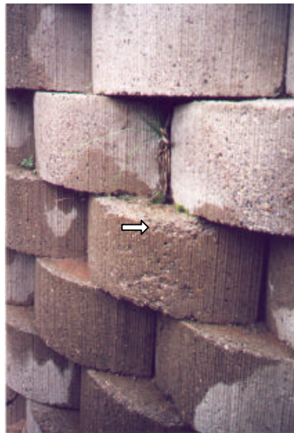
Medium-Severity Vertical Surface Scaling
