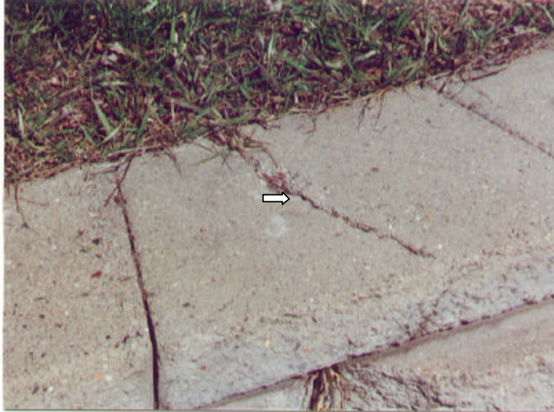
Medium-Severity Cracked Block
