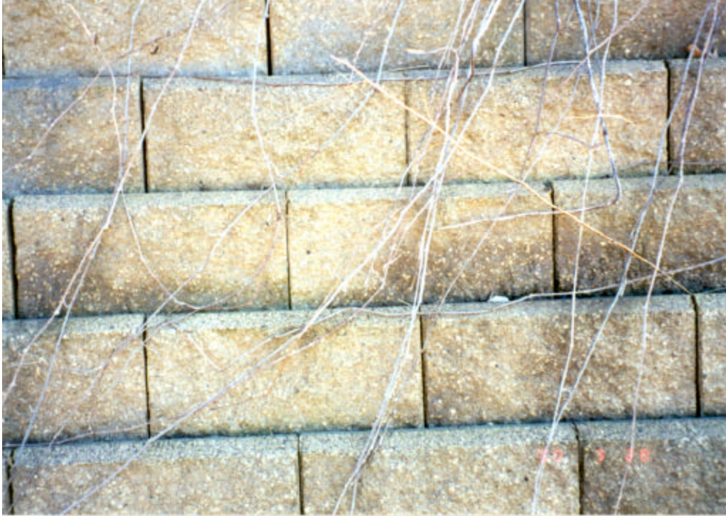
Figure 4.19. Photo of general condition of masonry blocks used in SCBRW subjectively rated as “fair”.
