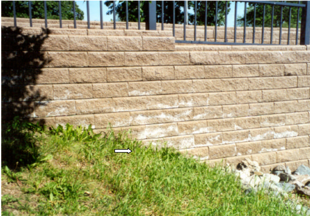
Figure 4.39. Photo demonstrating increased efflorescence in location near water runoff from sloped land.
