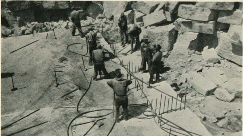
FIGURE 16.—Removing blocks from a quarry ledge by drilling and wedging. Quarry of the Breen Stone and Marble Company north of Mankato.
