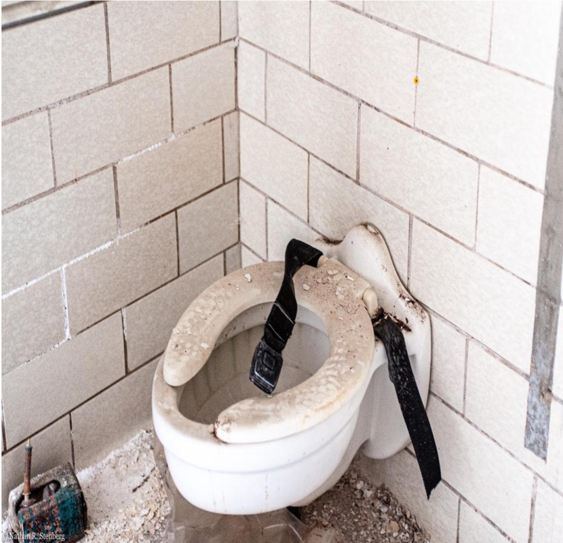
Figure 10: A dirt-covered, white-porcelain toilet with black restraints attached to it is affixed to a dirty, white-tiled bathroom wall in the PSSH's Infirmary building.
