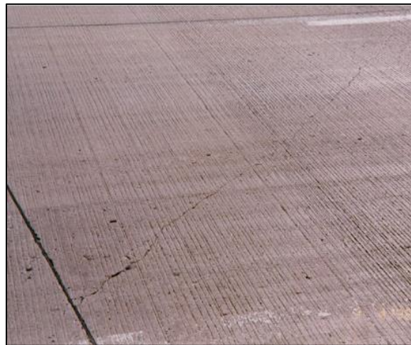
Figure 2.2 : Diagonal cracking (Harrington et al., 2018).
