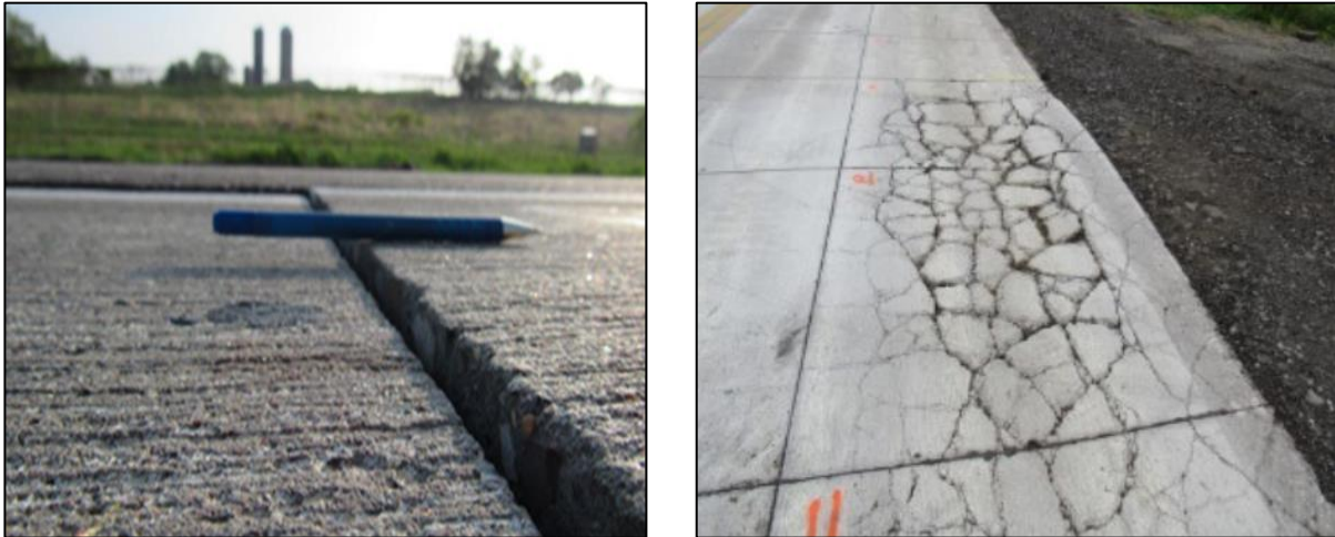
Figure 2.3: Joint Faulting in thin pavement (left) and slab shattering in ultra-thin pavement(right) (Barman et al., 2021).
